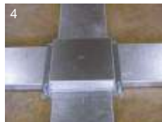
4 Fasten the trap frame, side blanks & ensure all the ductings and junction boxes are secured
